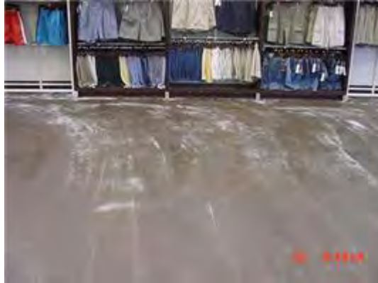
Whitening of sealer is often caused by applying it to a wet surface.
