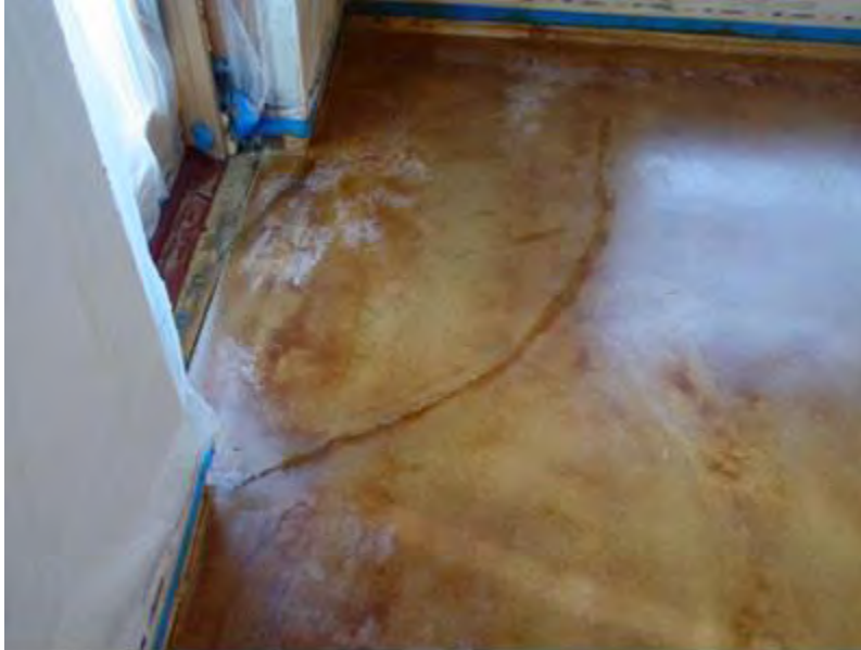
Water that condensed on a stained concrete floor by a cold doorway caused the sealer to white out in that area.
